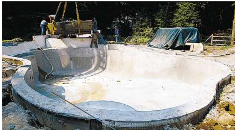
The 44,000-pound rock will be part of the Elfers family’s new swimming pool.
